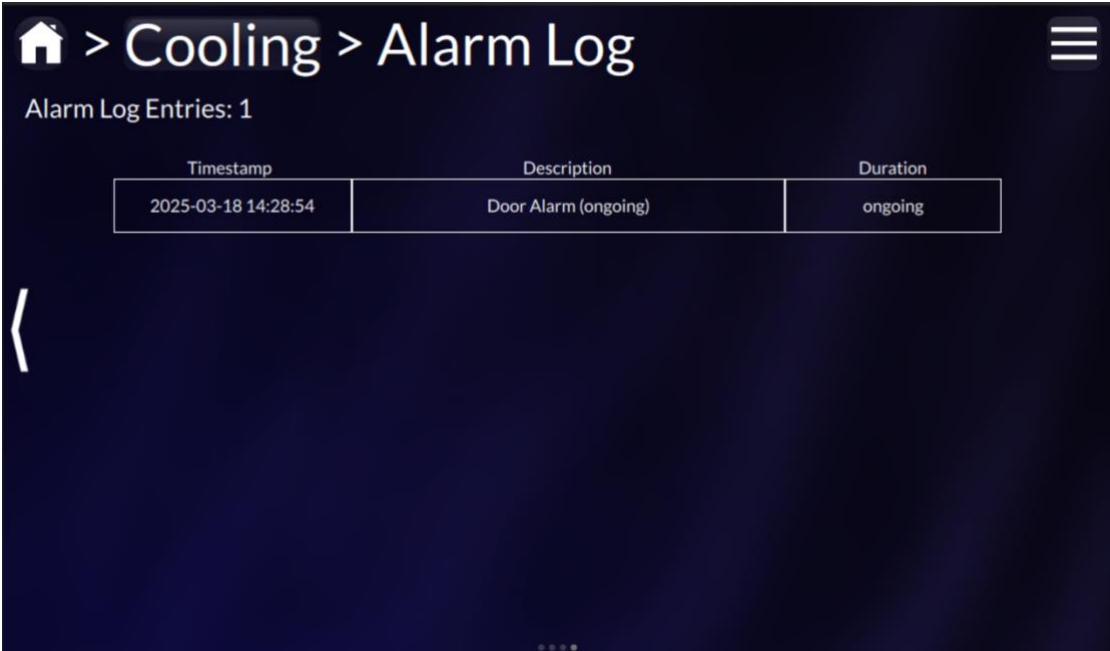
Figure 5-7 Alarm Log screen
